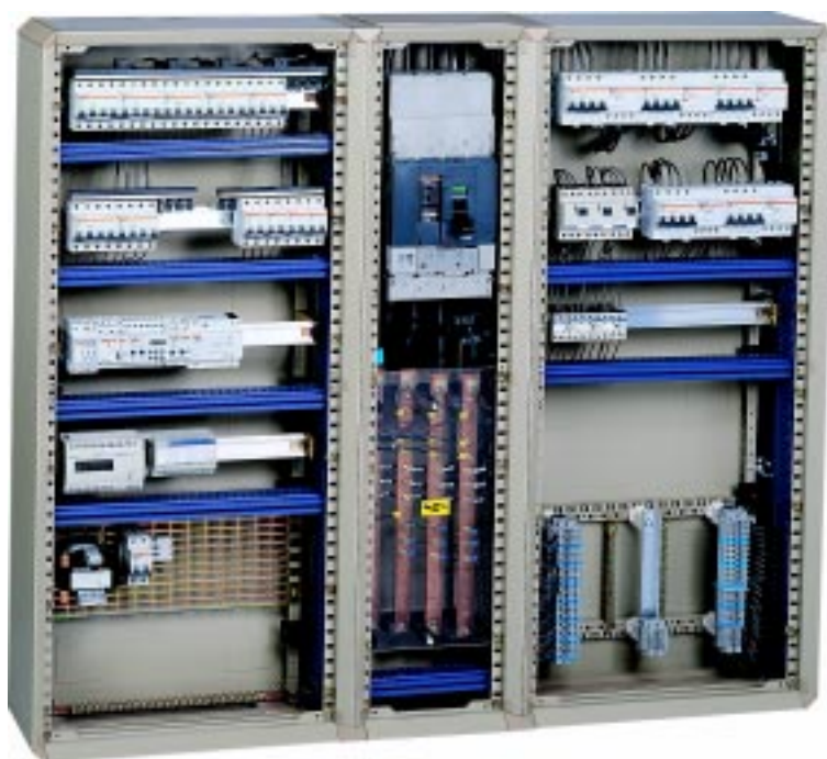
Top connected Compact NS400 used as incoming unit
