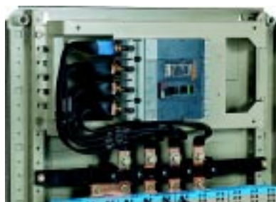
Incoming unit on a 250 A switchboard
