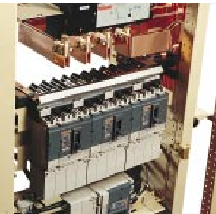
The auxiliary wiring is run in trunking.
