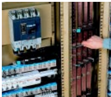
Complete access to points of connection.
