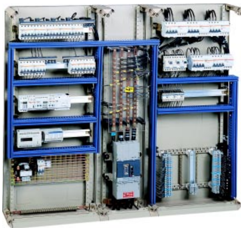
Bottom-connected Compact NS400 used as incoming unit. Distribution block in the duct.
